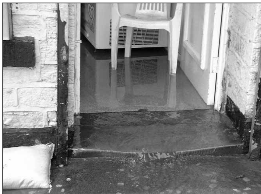
Figure 1.3 Example of property damage due to storm sewage flooding (courtesy Pennine Water Group)
